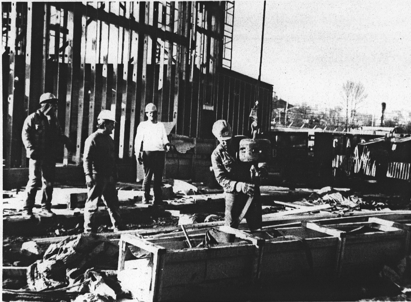
Much of the construction on the Navy's Stapleton home port is 70 percent complete, with about 100 navy personnel living there. The first two ships are scheduled for an August arrival. Of the $206 million contracted for construction, $167 million worth has been already built. Included in that figure are about 126 homes, out of 400 housing units to be built, finished and there are families now residing there. Completion of housing, a maintenance warehouse, the primary pier and other crucial facilities for the base will continue to be constructed because a construction moratorium was announced after contracts for that work were signed.
