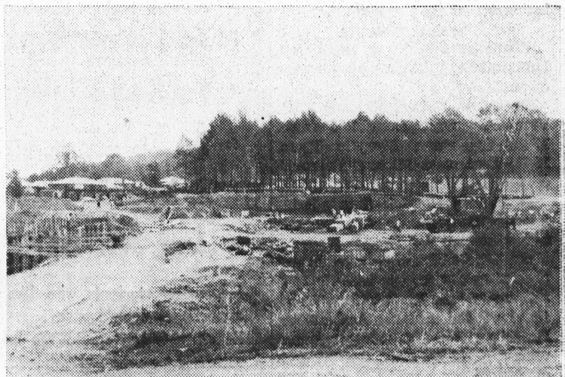
Construction continues at Sunnyside campus. Left photo is of building foundations. Clove Lake Expressway is in the background. Grove of trees on the right will be part of new campus.
