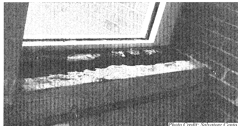
A piece of the windowsill is missing and pollutants are sneaking through in 3N.
