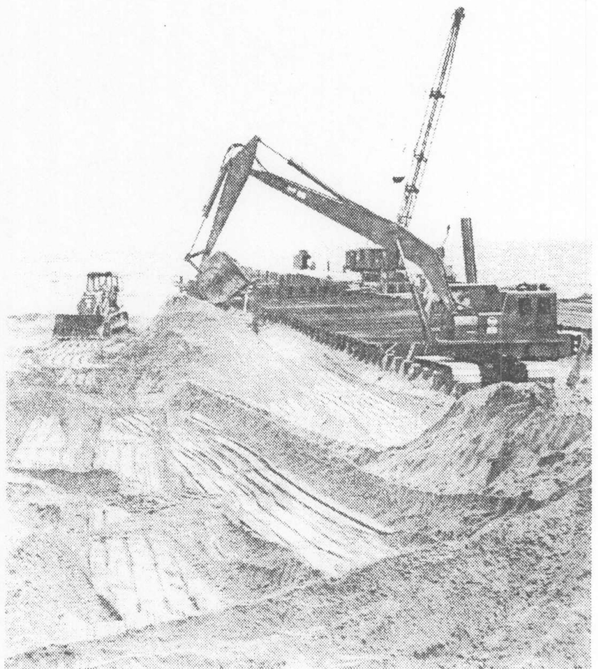
This sewer outfall under construction at the foot of Seaview Ave., Ocean Breeze, will connect with a massive network of new sewers in the Grasmere-Dongan Hills area. Flooding, a constant problem in the Board 2 area, should be eased.
