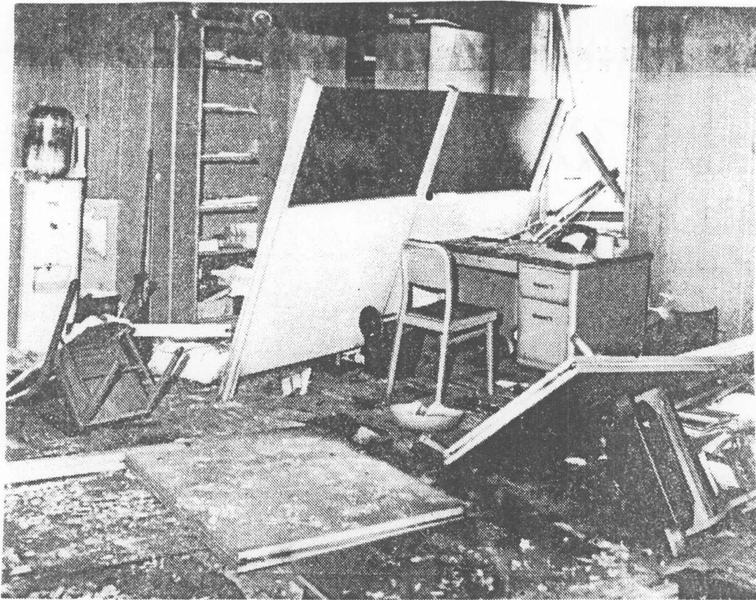
The charred interior of an office in the Dumont Ave. building.
