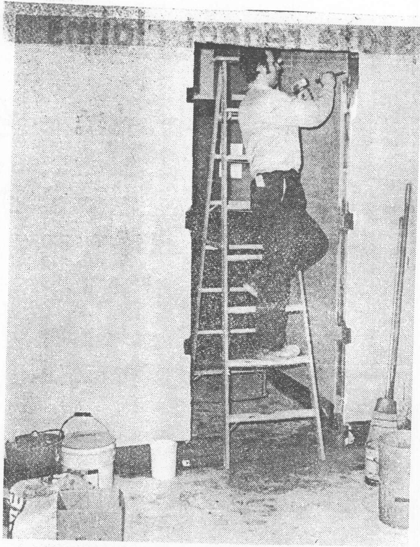
A workman frames out a doorway area in the new office complex of Assemblywoman Elizabeth Connelly at Willowbrook Developmental Center. The Democratic lawmaker is scheduled to move from her West Brighton office next month.
