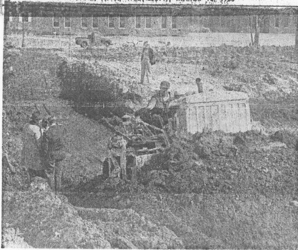
WILLOWBROOK PROJECT —Workmen begin excavating for foundation of new infirmary at Willowbrook State School. The one-story structure will cost approximately $800,000.
