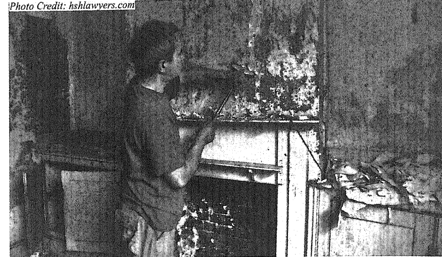
A man painting a wall while being exposed to Asbestos.
