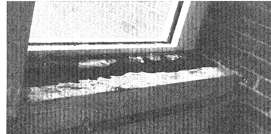
Photo Credit: Salvatore Cento A piece of the windowsill is missing and pollutants are scouring through in 5N.
